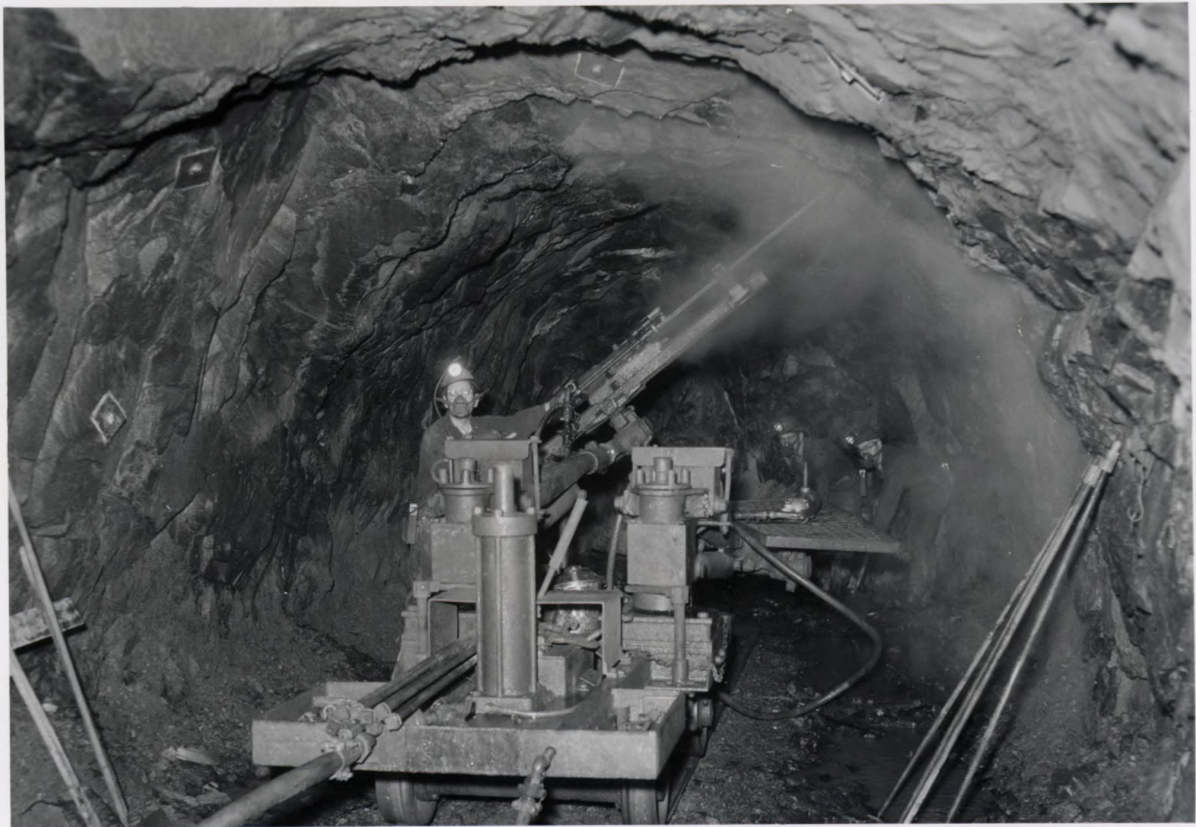
Drilling holes for installation of rock bolts in 9th Level drift heading.
