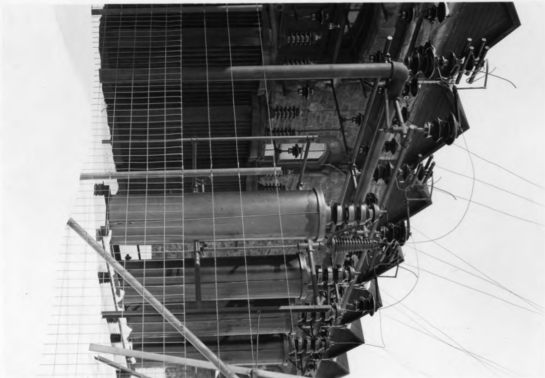
Plate No. 203 - Outdoor Transformers - Brownstone Substation
