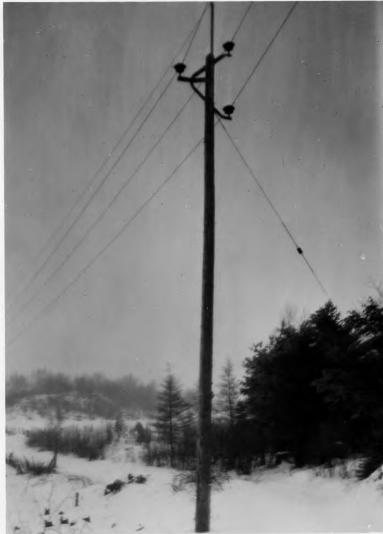
Plate No. 218 - Wood Pole on New Line from McClure Plant to Maas Mine.
