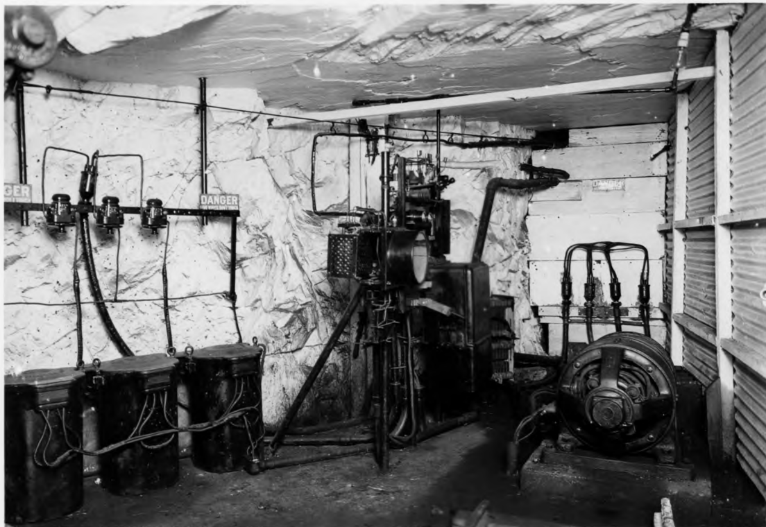
Plate No. 211 - Charging Set for Storage Battery Locomotives - Republic Mine
