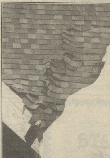
Ice buildup is causing the shingles on the dome much havoc. (Andy Gregg photo)
