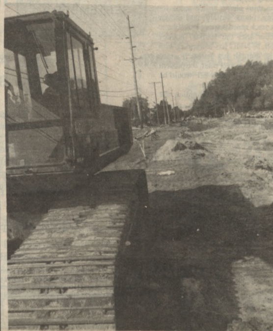
NMU's campus isn't the only place under construction in Marquette. North Presque Isle Avenue has been under construction for most of the summer. (Andy Gregg photo)
