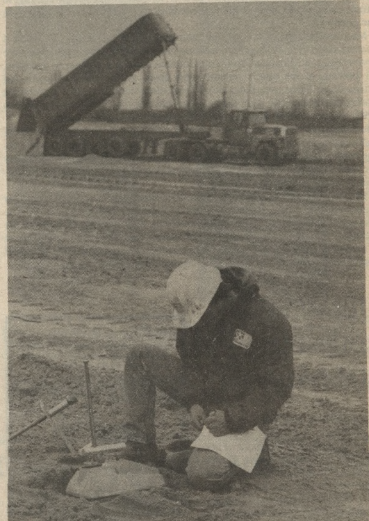
A construction worker measures the compaction level of the soil where the multi-million dollar sports dome will stand. (Kate Vinson photo)
