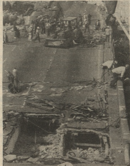
The emergency rescue efforts were abandoned yesterday when the collapsed Highway 880. The bodies of the remaining victims will be removed when they are reached during the clean-up effort. (AP photo courtesy of the Mining Journal.)
