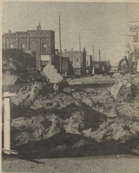
Third Street construction is expected to be completed in November. (Photo by Kim Kelper)
