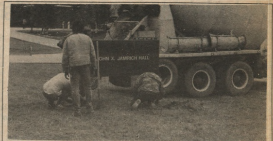
Cook Sign and Design employees working on the installation of the new Jamrich sign last spring. (North Wind file photo)
