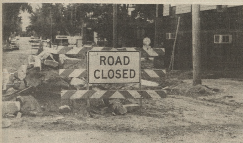
Third Street renovations, which began last spring, continue and have reached Hewitt Street. Pictured is Third Street at Park Street. (Kim Keiper photo)
