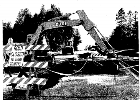
City crews replace the sewer line on Lake Street, running north from Main Street, after discovering that some 320 feet of old crockery sewer had collapsed. In addition, workers had to replace the Main Street manhole, which had also failed. (Pioneer-Tribune photo)
