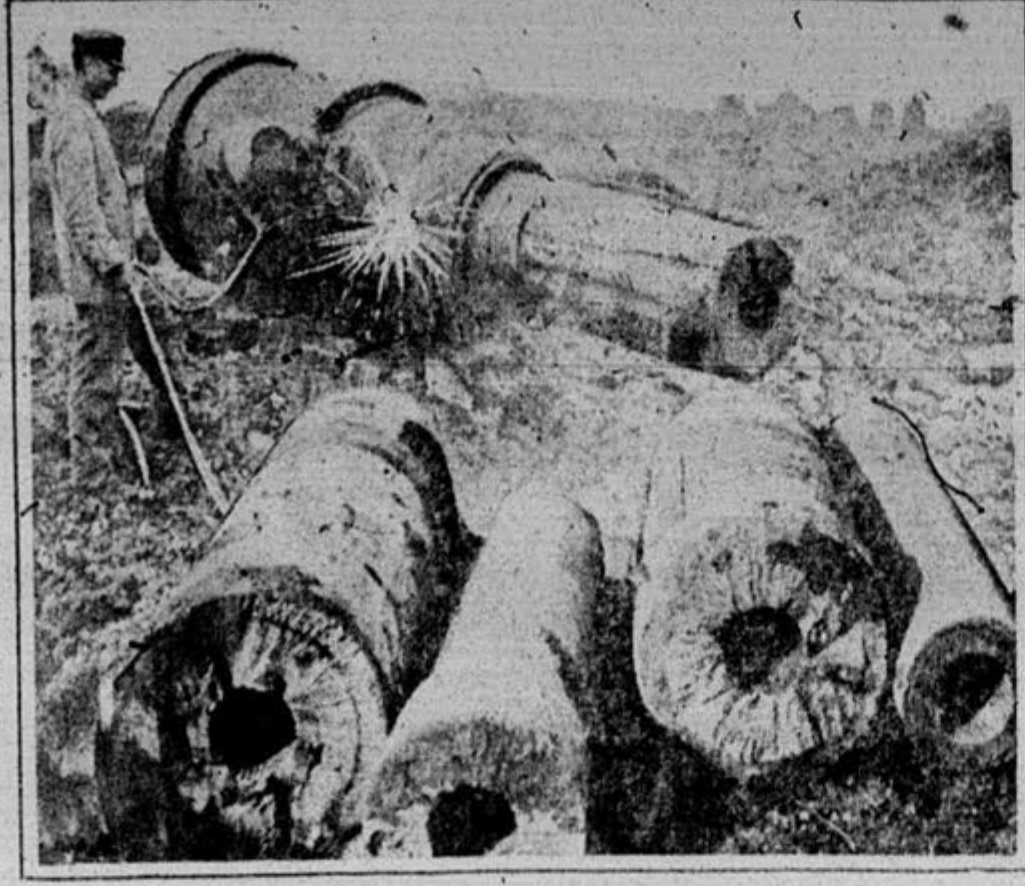
In accordance with the terms of the Versailles peace treaty the great German fortresses at Kiel is rapidly becoming a junk pile. Remains of some of the powerful 15 and 24-c. m. guns are shown in the foreground. The workman is using a metal-cutting torch to destroy the other monster.
