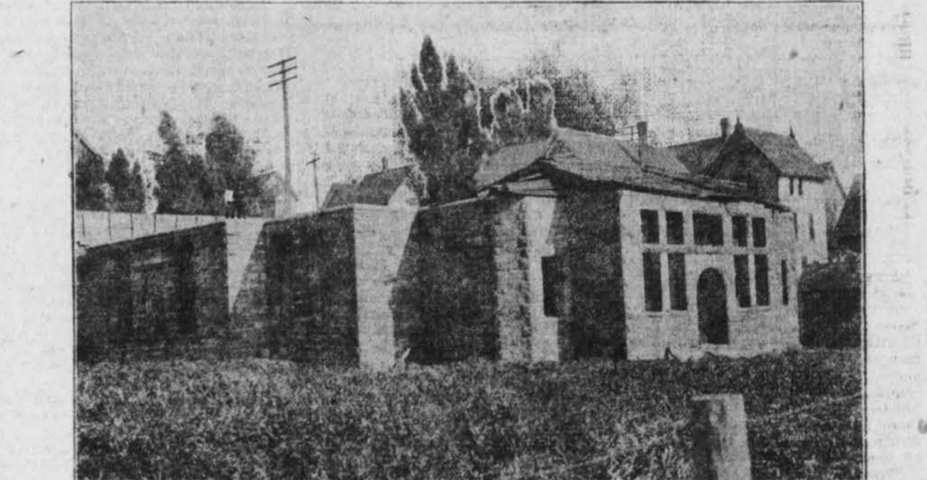
Foundation for the eight-family flat to be erected by the National Finnish Brothers' Temperance association as seen from York street.
