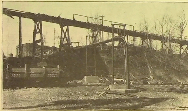
FIG. 6.—EXPANSION OF THE TANGENT TAKEN UP WHERE IT EMERGES FROM THE BURIED BOX. LONG HANGERS ARE NEEDED, AS A TRAVEL OF 12 OR 13 IN. IS REQUIRED.
